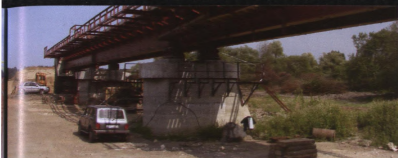
Railway bridge at Shchuch'ye crossing the Miass river between the chemical weapons destruction facility and the storage site.
