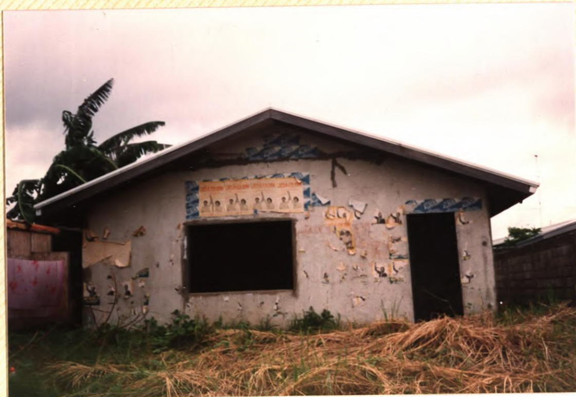
No. 72. An unfinished house constructed with a system of pre-cast concrete panels erected on site.
