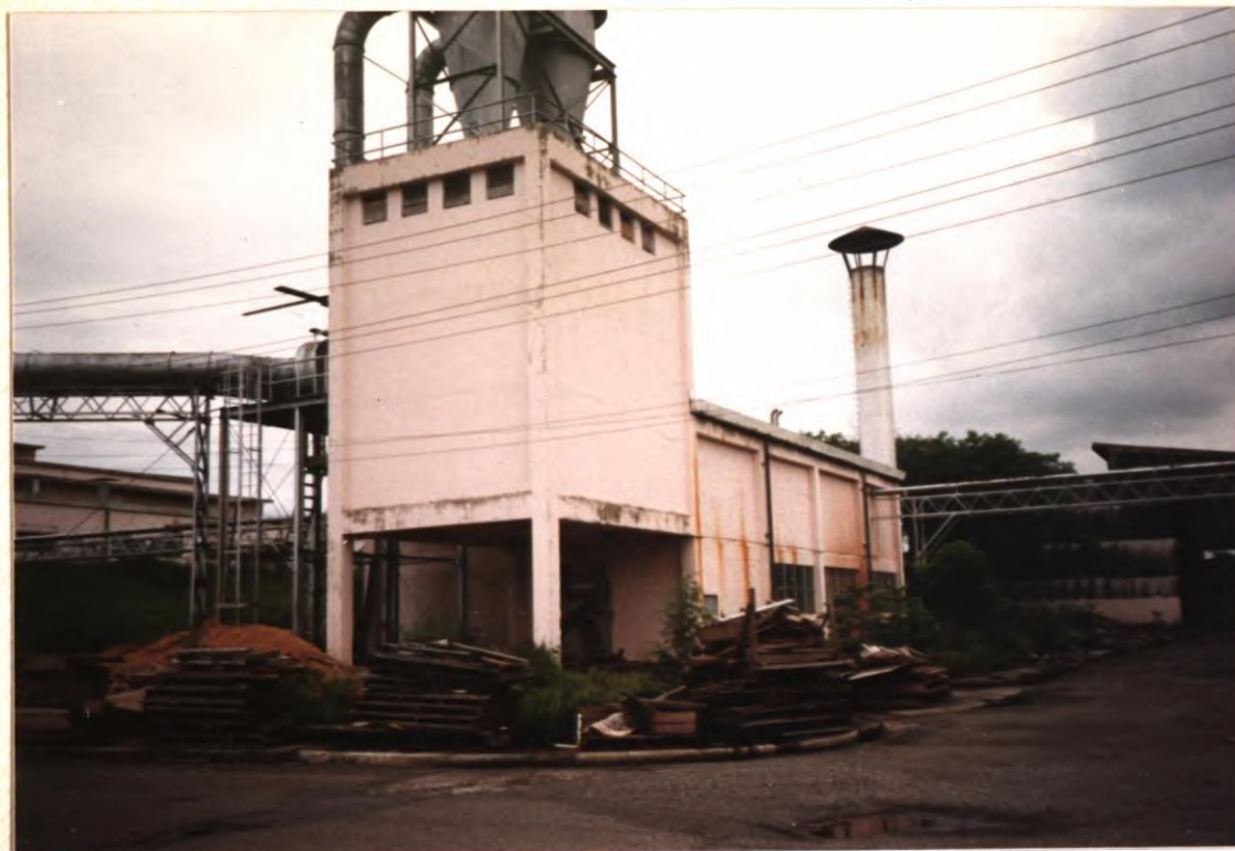
No. 25. Boiler house providing steam to lumber dry kilns, wood preservation and lightweight concrete curing.
