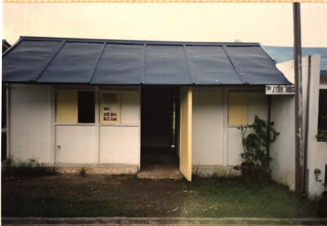
No. 40. "Zytec House" front entrance showing sheet metal roof, 2x2 panel framing and wooden shutters on windows.
