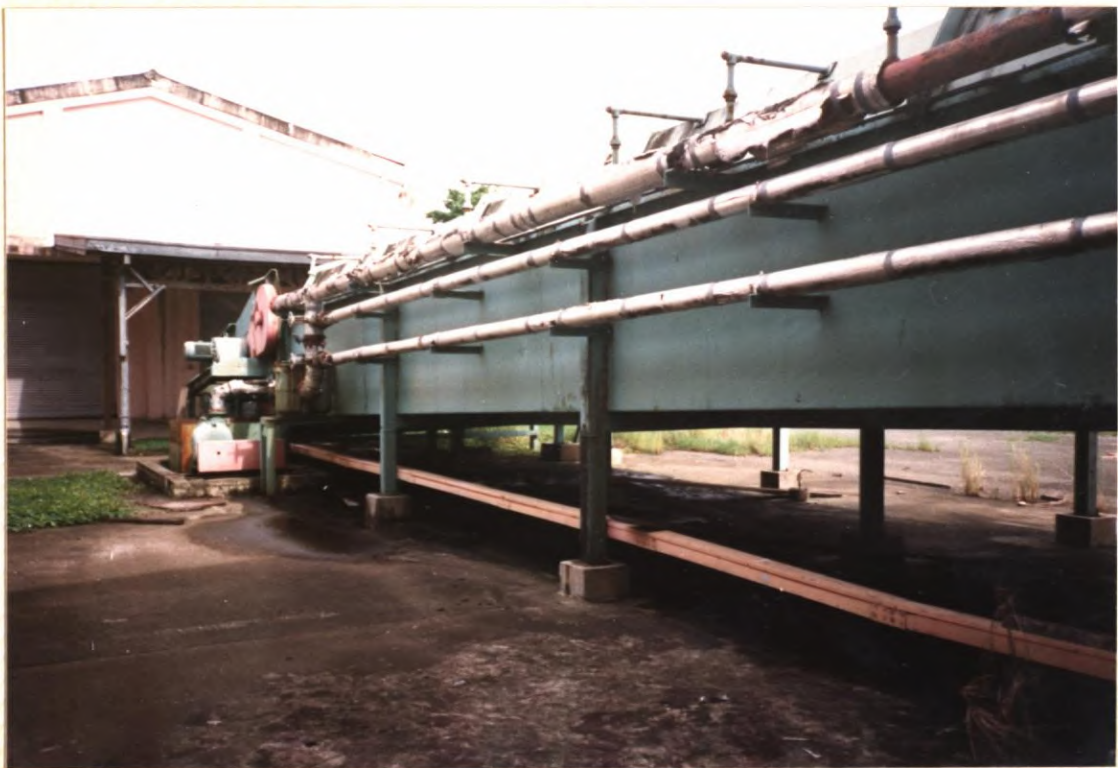
No. 14. OSB log infeed conveyor.
