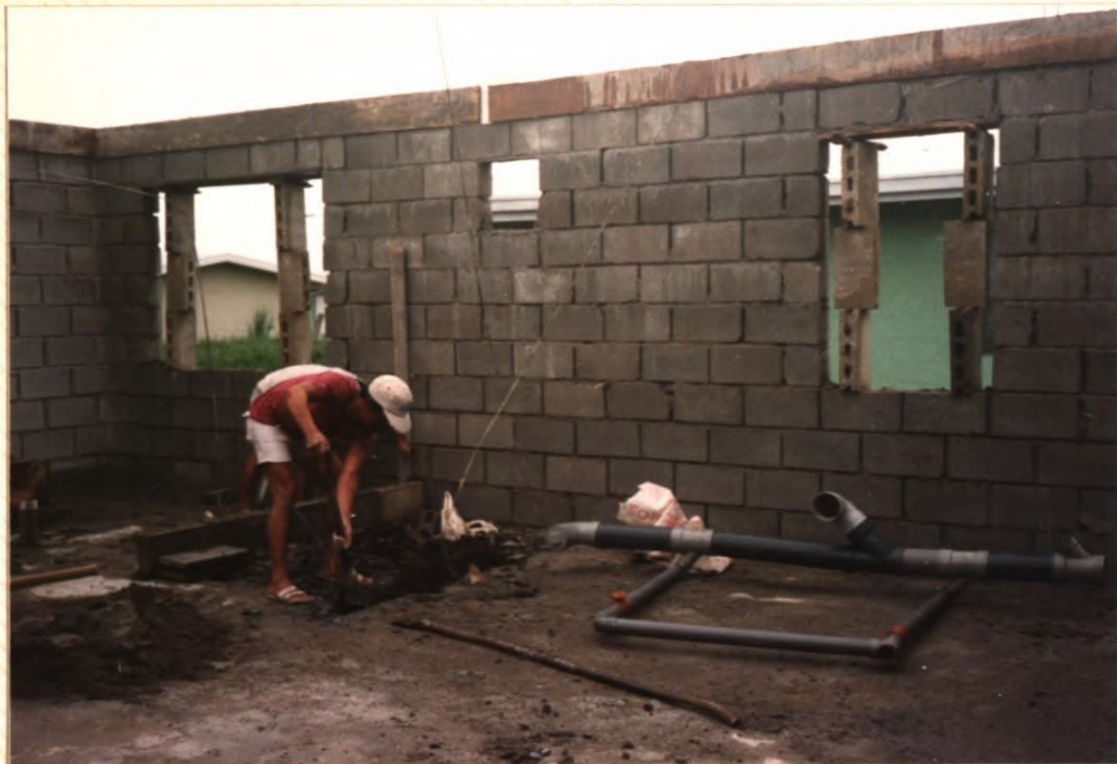
No. 62. Installing toilet plumbing. Note window header supports while concrete is curing.
