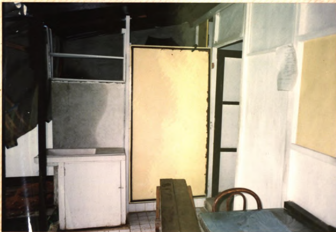
No. 41. Right side of covered back porch on Zytec House showing kitchen sink. Shower stall and toilet are behind yellow door.
