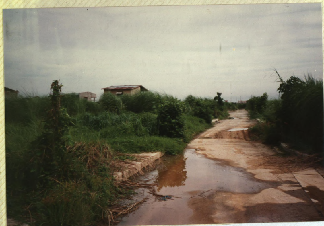
No. 56. Street in site and service subdivision showing lack of maintenance.
