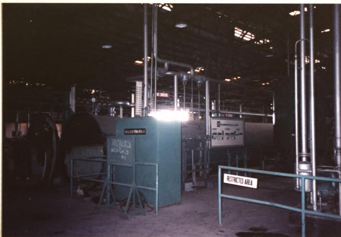
No. 21. Pressure treatment vessel with door open.
