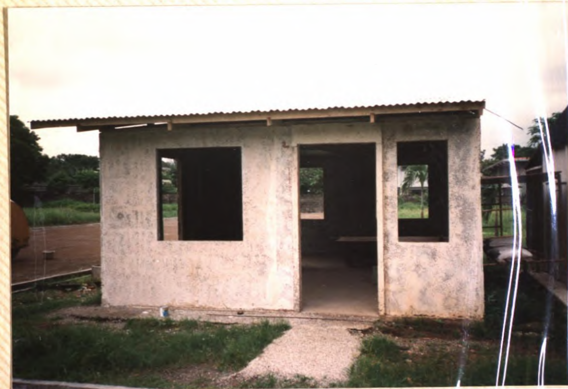
No. 43. The "MKL-33 House" front entrance. Note corrugated sheet metal roof and semi-finished state of construction.
