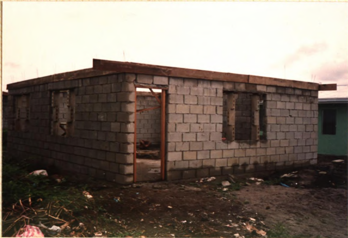
No. 61. This series of photographs, Nos. 61 to 69 will show the steps in the construction of a typical hollow-block house.
