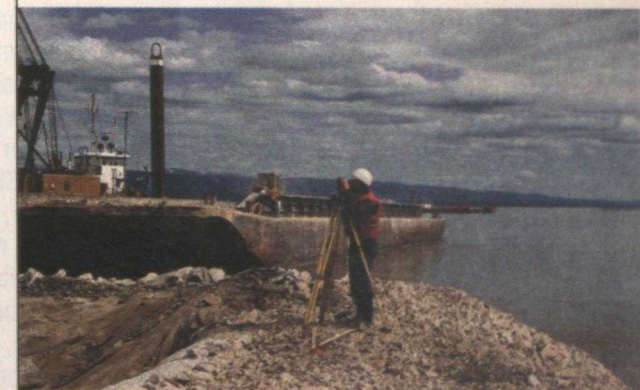
Engineering surveys for ports and harbours construction are among the services of Usher Canada Limited.
