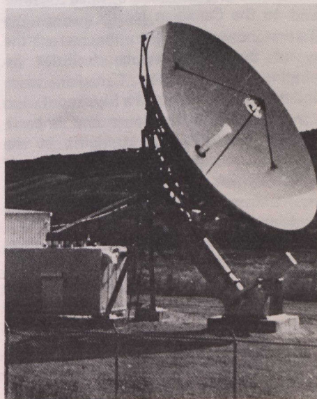
A receiving dish at Telesat Canada's network television station in Qu'Appelle, Saskatchewan.
