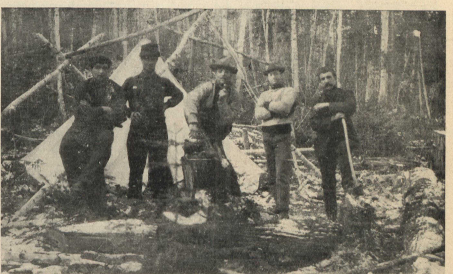
The Road-Cutters in the woods of Northern Ontario are busy chopping out the way for the "iron horse" on the Transcontinental Railway.
