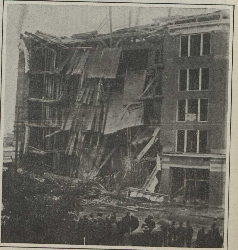
An apartment house in Calgary became a mass of debris on August 26. Fortunately this phenomenon is of rare occurrence even in a land of headlong haste in building.
