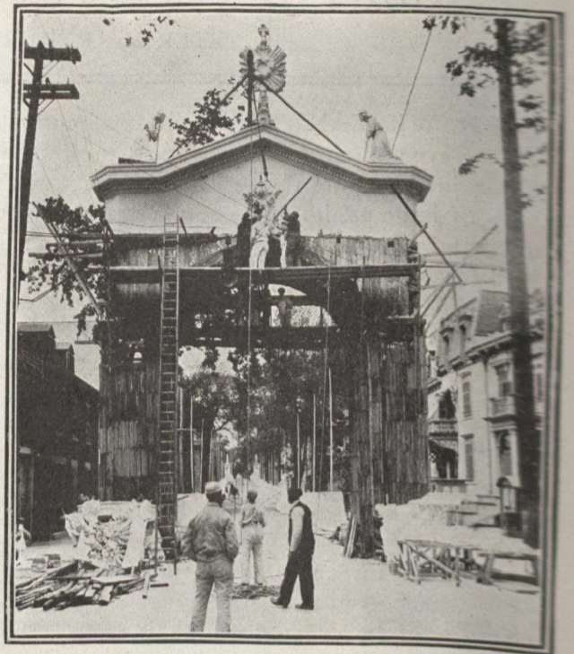
Building central arch on St. Hubert Street. Lath and plaster are the main materials used. The figures and decorations are cast separately and then placed in position.
