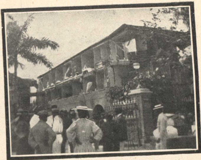
Right Wing of Myrtle Bank Hotel, the walls of which fell into the Courtyard.
