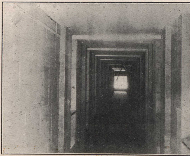
Corridor in Christian Bros. School, Longueuil, P.Q., showing SACKETT PLASTER BOARD before "FLAWLESS" HARD WALL PLASTER was applied.
