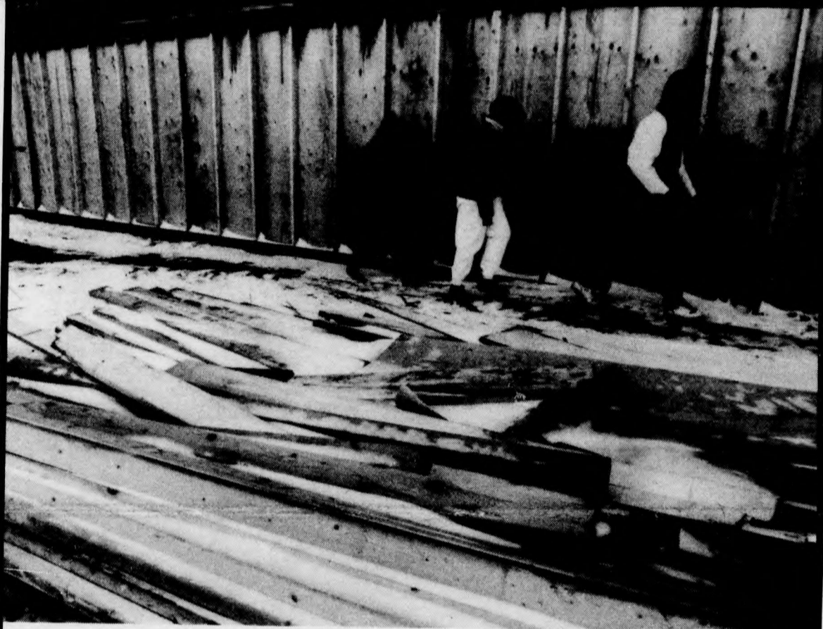
Abbey Road à la York . . . construction begins on the Entry Pavilion east of Ross
