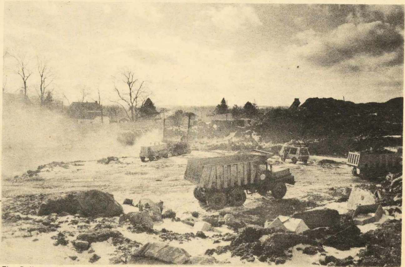
The Dalhousie Sports Complex is underway, but residents have complained of home damage due to the blasts.
