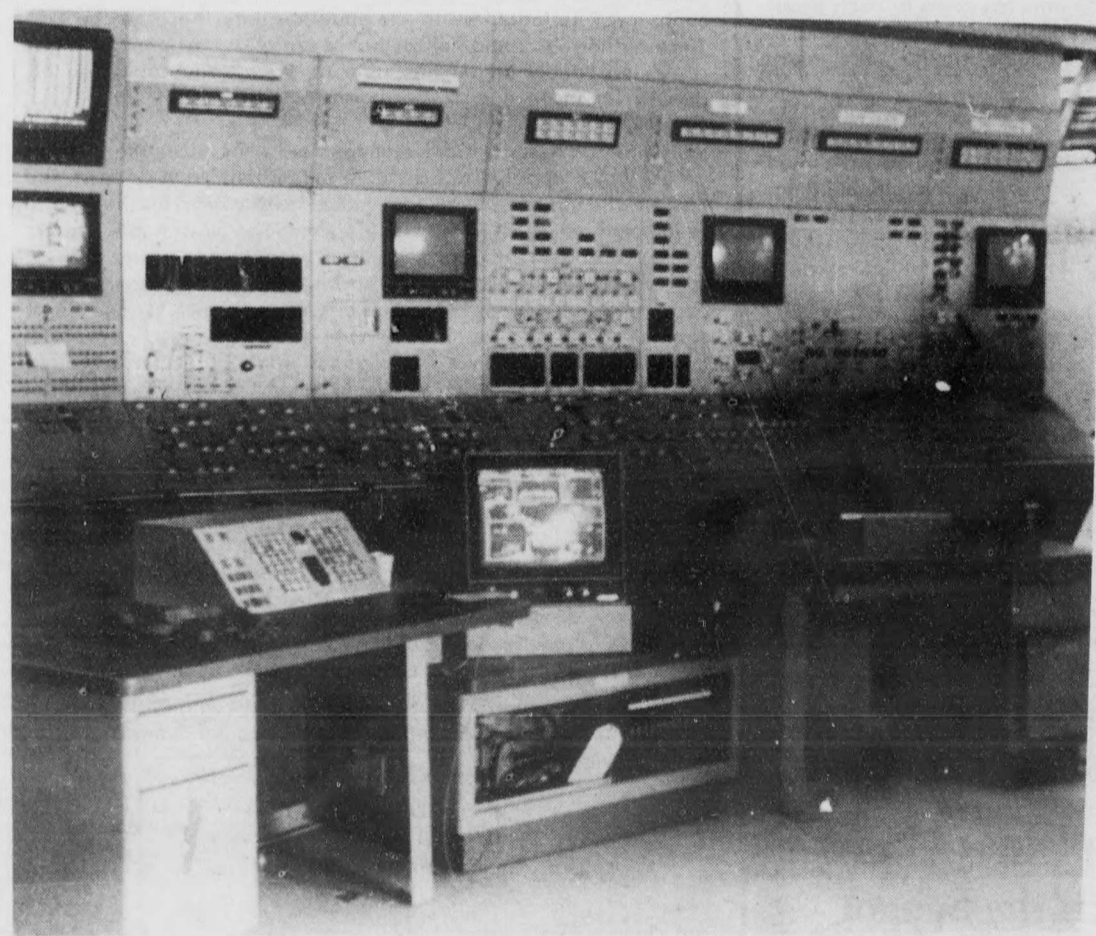
The main control room at Lepreau.
