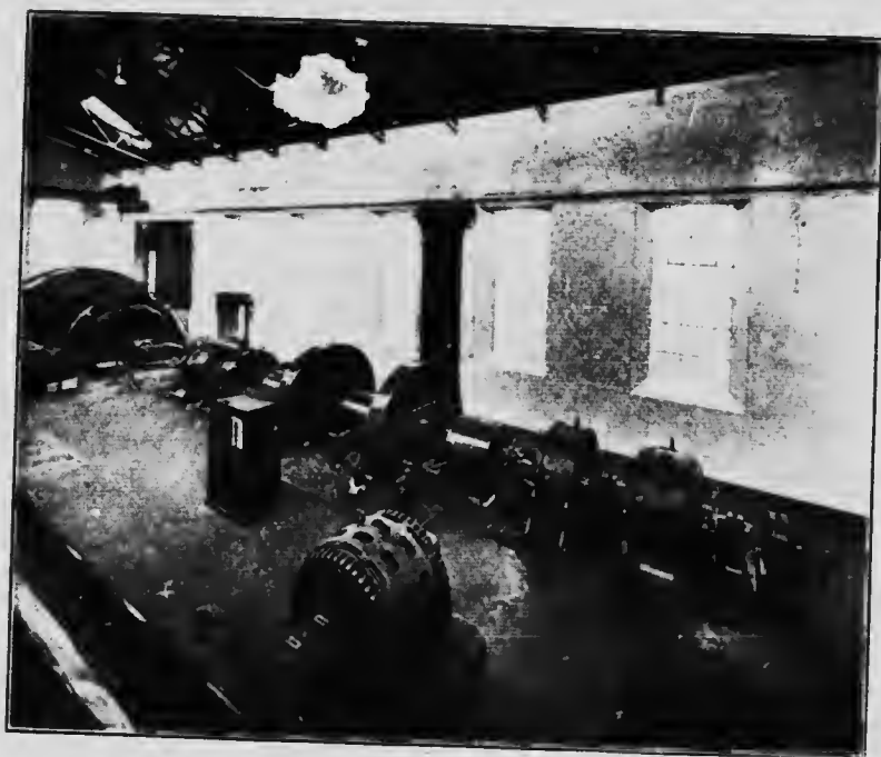
Fig. 11 Ilgner flywheel motor generator set supplying the two winders at the Markham Steam Coal Company. Consists of two flywheels, two variable voltage D.C. generators driven by two three-phase motors, each 660 horse-power, 510 to 590 r.p.m. on 6,600 6,000 volt, three-phase, 50 cycle circuit.
