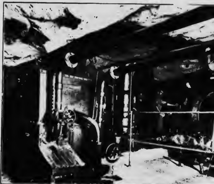
Fig. 29 Underground three-phase hoist, showing liquid controlling resistors.
