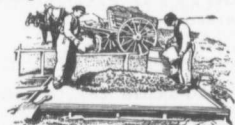
THE mixing and placing of concrete is simple, and is easily learned. No elaborate tools are needed.
