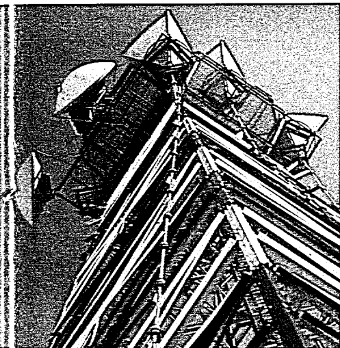
Digital Microwave . . . One of the towers in TELECOM CANADA's dual transcontinental chain of microwave radio routes. A substantial portion of this network operates using digital transmission techniques.
