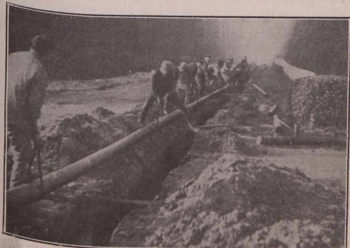
Fig. 2.—Stretch of pipe being lowered into trench after pipe has been welded above ground.
