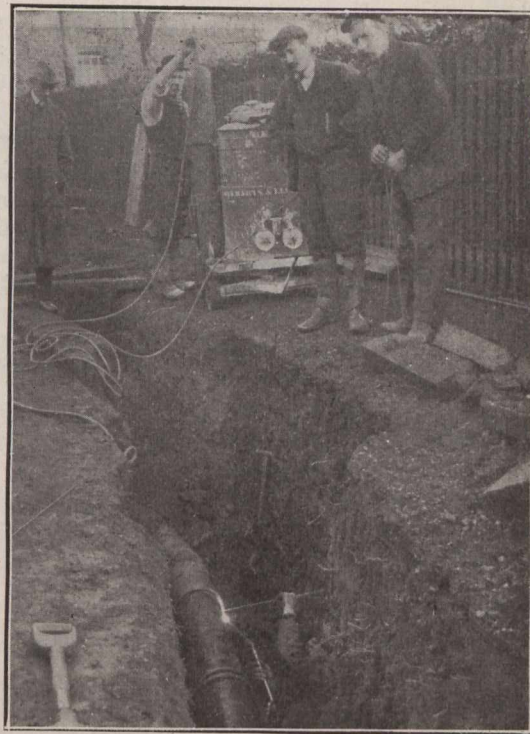
Fig. 3.—Welder at work in position where it has been impossible to turn pipe so as to keep welding portion at the top. A recess was made to allow the welder sufficient space to work all around the joint.
