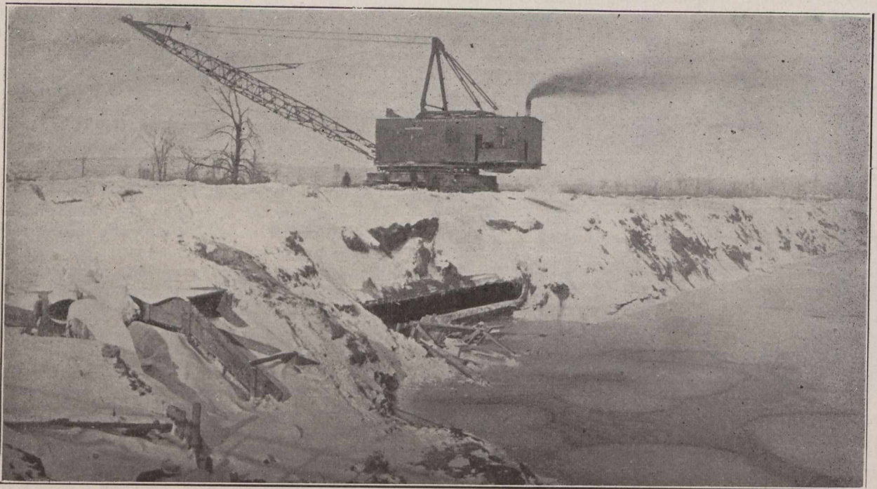
Fig. 3.—Montreal Waterworks Conduit Break as it Appeared on December 27th, 1913. (Drag line excavator has been moved up from point of operation at extreme right of photo, to be used in excavating the earth around the break).
