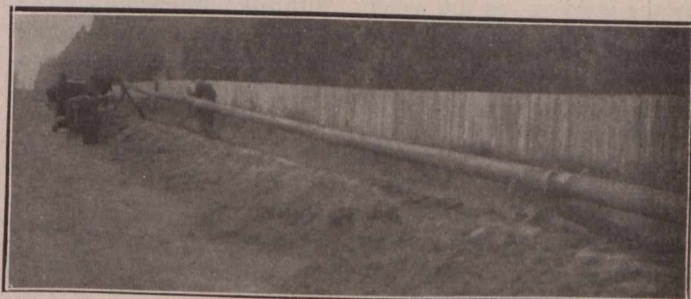
Fig. 4.—Six-inch pipe welded on trestles, then settling by its own weight into trench.
