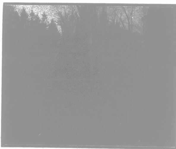
Cut 2.—Underdrainage Needed. The photo from which this engraving was made was taken the same day as that reproduced in Cut 1. This piece of road is just north of the other, and until the other was underdrained this was much the better of the two.
