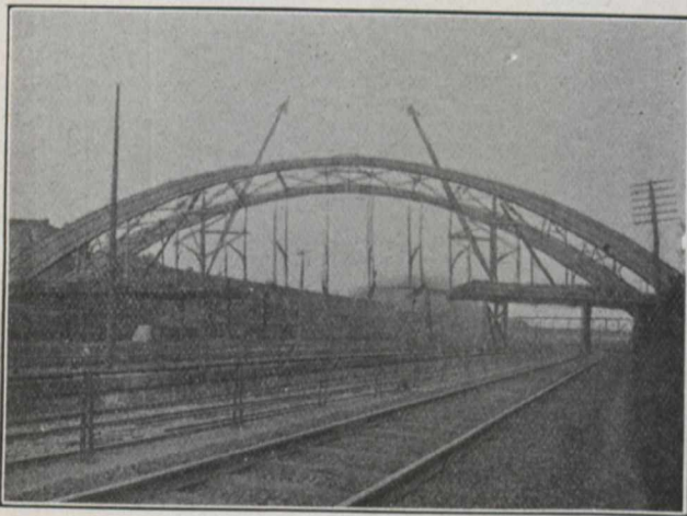
Forty-Second Street Bridge, Philadelphia, Pa.—Steel Arches Completed and Suspenders and Floor Beams in Place.
