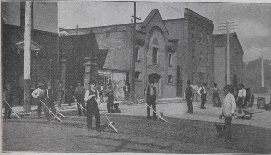
An Elastic Filler—Pouring "Pioneer" Filler Asphalt into brick paving joints, London, Ont.
