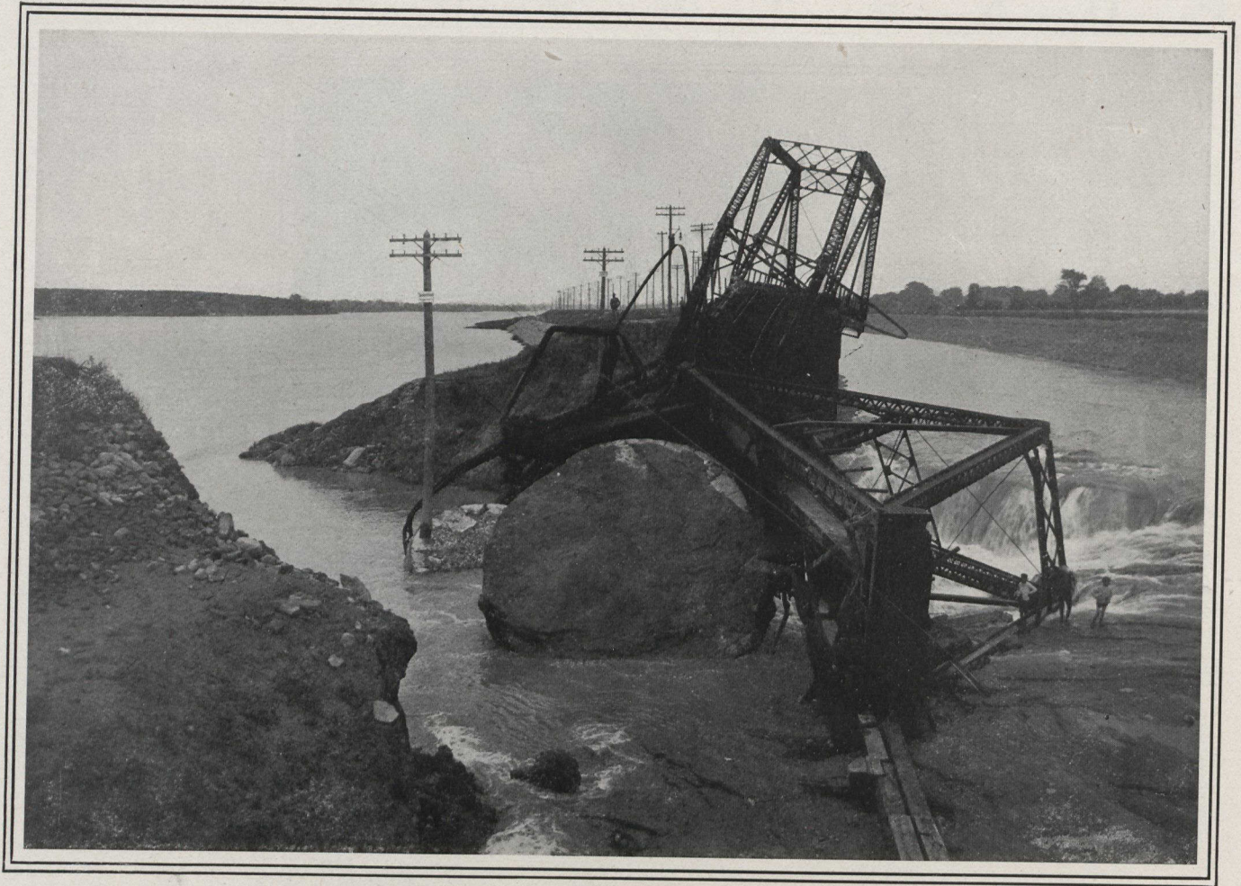
VIEW OF THE WRECKED BRIDGE OF THE ONTARIO AND NEW YORK RAILWAY, WHICH WAS CAUSED BY THE BREAK IN THE CORNWALL CANAL.
