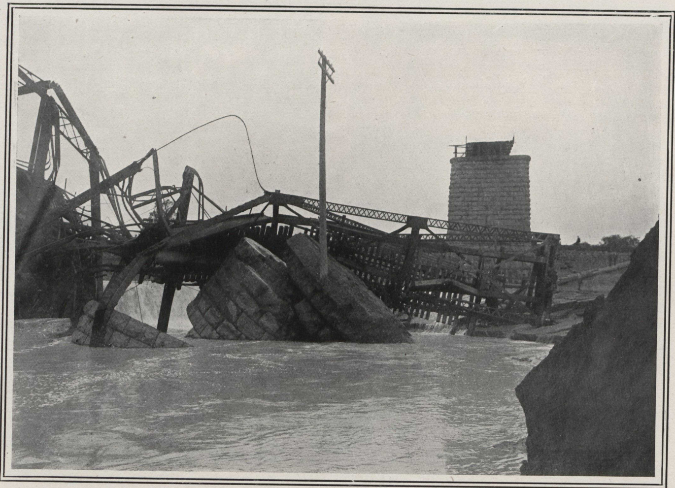
ANOTHER VIEW OF THE WRECKED BRIDGE, SHOWING THE COLLAPSED PIER IN THE FOREGROUND, AND THE COMPLETELY DEMOLISHED SUPERSTRUCTURE.
