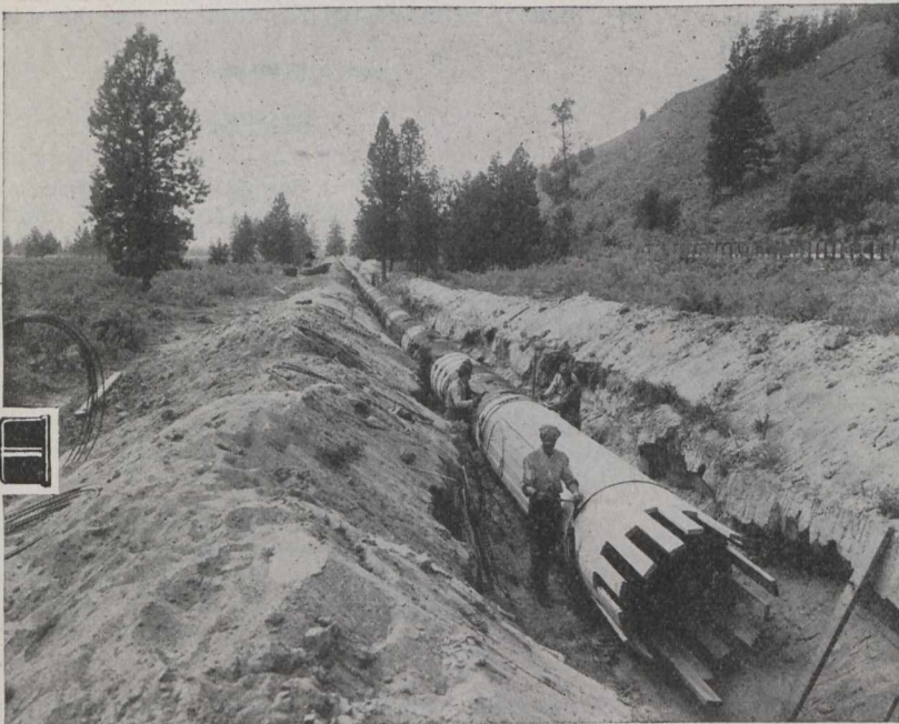
48 in. CONTINUOUS STAVE LINE.
