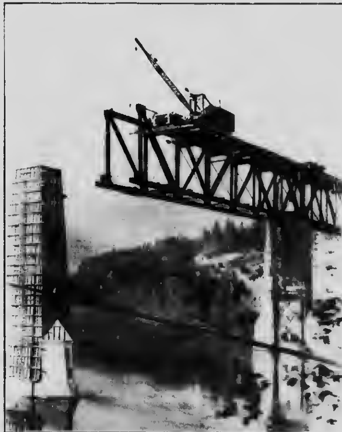
THE SKEENA RIVER BRIDGE, BRITISH COLUMBIA, GRAND TRUNK PACIFIC RAILWAY. THREE 100-FT. SPAN AND THREE 70-FT. SPANS. THE FORMER BUILT BY CANTILEVER METHOD FROM ONE END.
