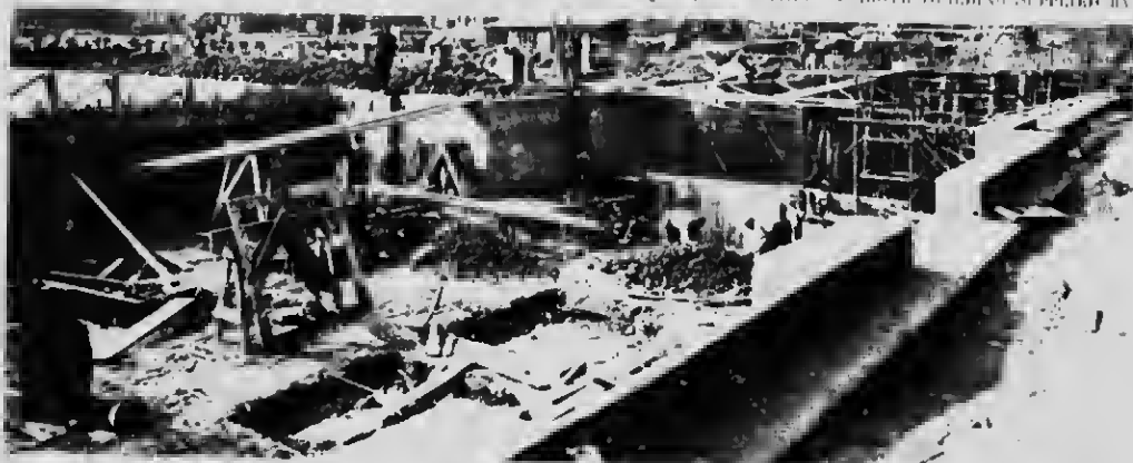
FOUNDATIONS OF TEN C.P.R. FREIGHT TERMINALS, TORONTO WATERPROOFING ON ABOVE FOUNDATIONS EXECUTED BY U.S.
