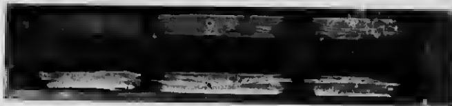
A TELEPHONE CROSS ARM TREATED WITH SOLIGNUM. Note how the penetration is all around the supply joints where it is most needed. Solignum takes the points of least resistance.
