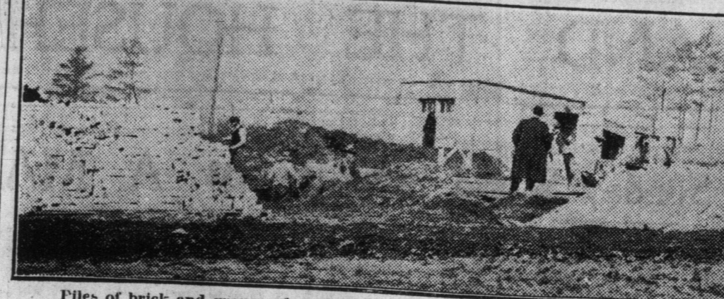
Files of brick and groups of workmen digging cellars and laying foundations are sure auguries of the approach of warm weather. A score of such indications mark the commencement of the building season in Glebe Manor.
