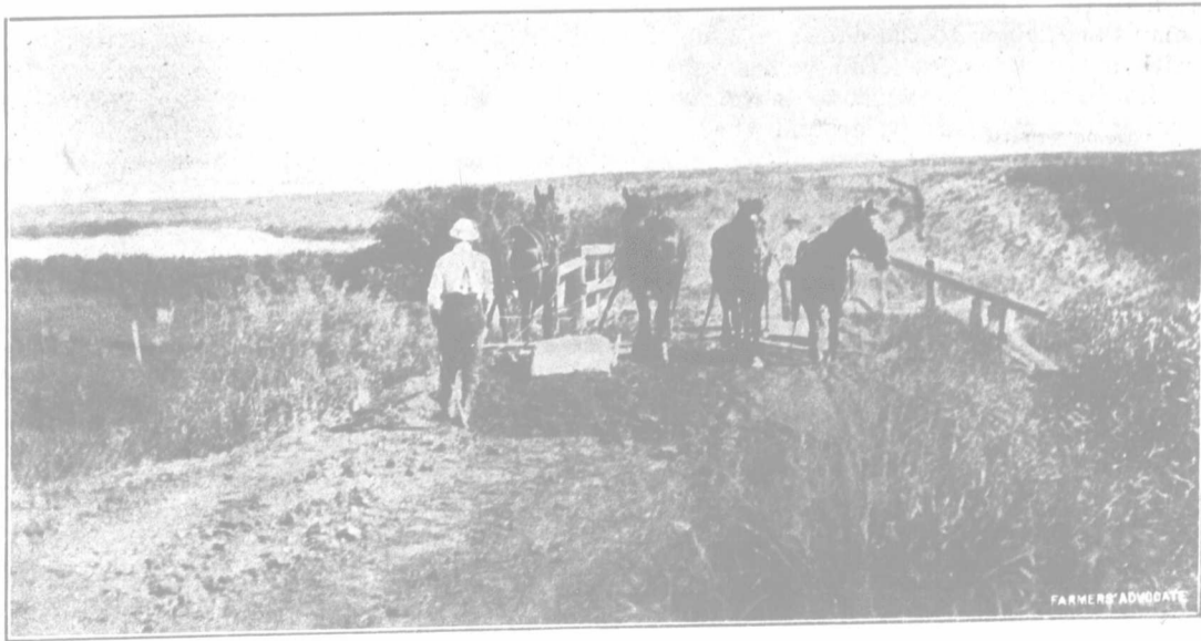
TEAMS AND SCRAPERS ATTEMPTING TO REMEDY DEFECTIVE WORK DONE BY STATUTE LABOR
