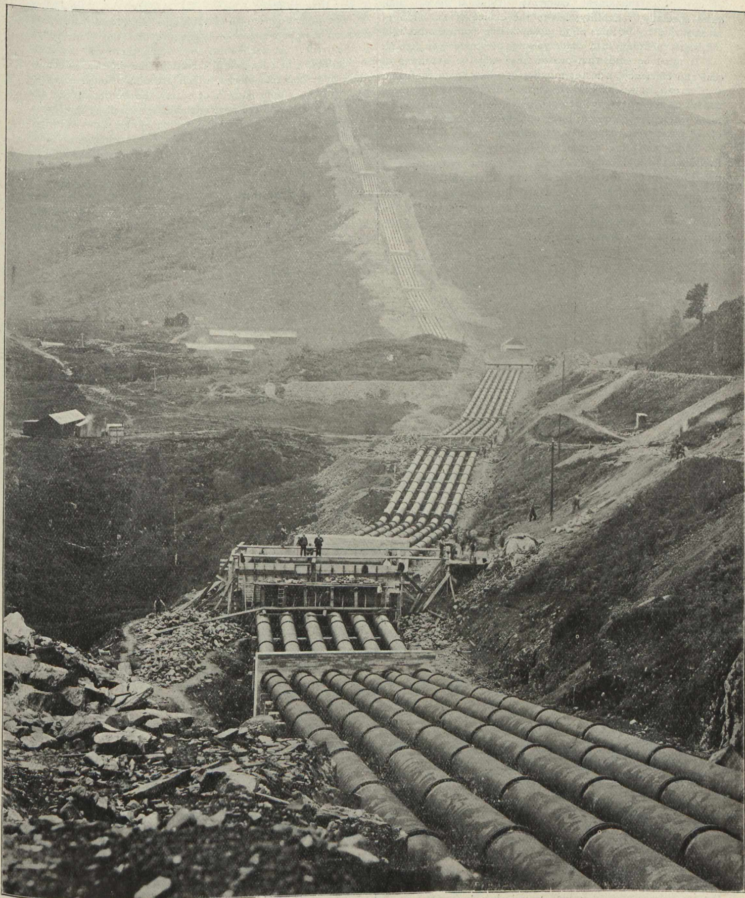
LOCH LEVEN POWER PLANT
