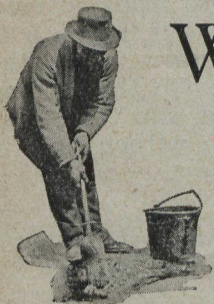
The hole to be patched is cleaned and the bottom and sides are painted with "Tarvia-KP."
