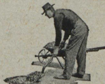
The mixture of "Tarvia-KP," stone and sand, is placed in the prepared hole.
