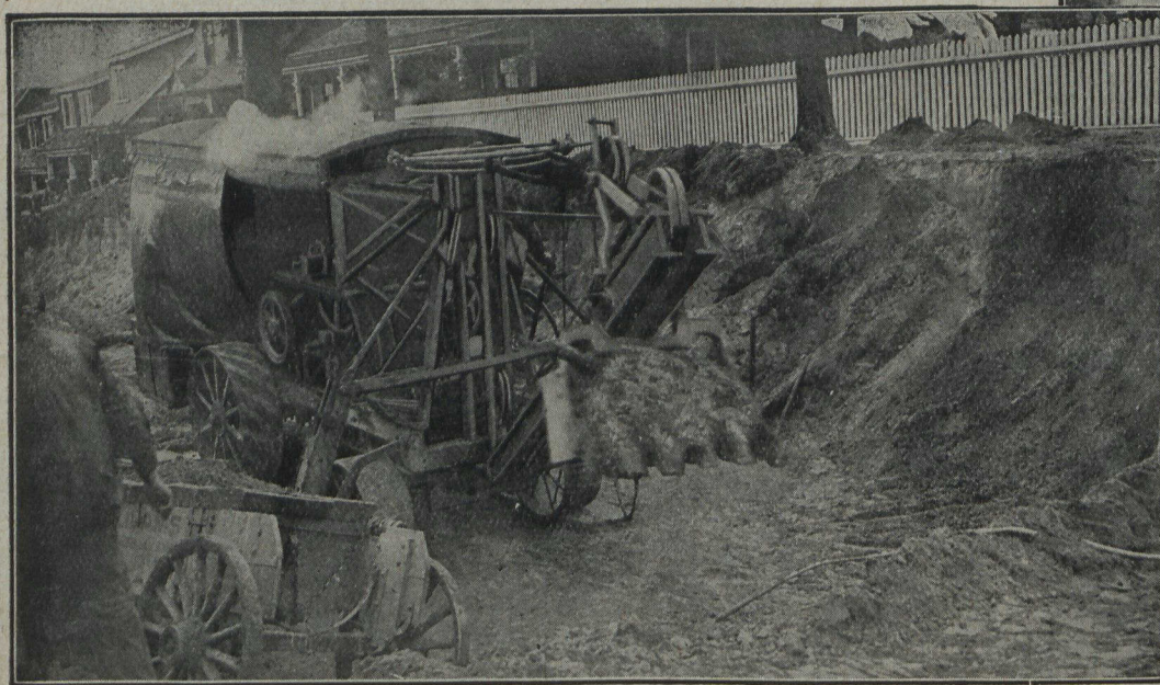
Keeping the dump wagons moving in a Toronto grading job with the Keystone.
