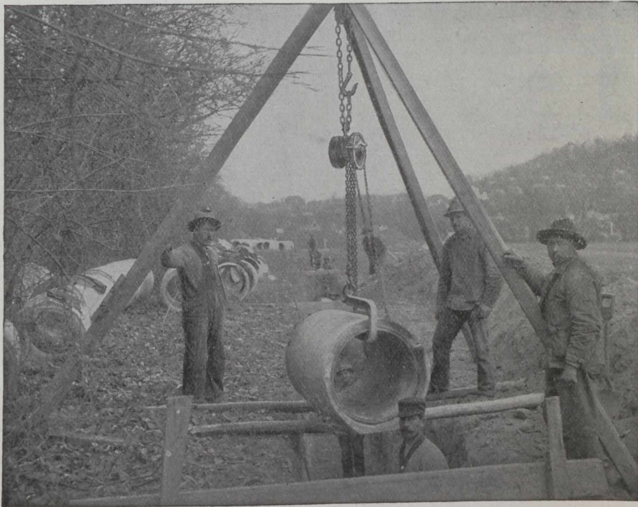
A Triples Block hung from a temporary rigging and used for laying pipe.
