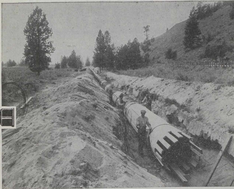
48 in. CONTINUOUS STAVE LINE.
