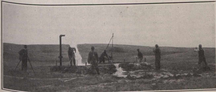
View of Well Showing Measuring Weir.
