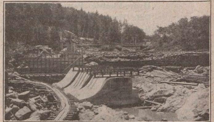
PORTION OF SLUICWAY SECTION OF DAM, SHOWING THREE OF THE FOUR ROLLWAYS
