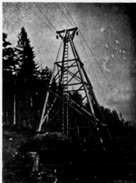
Recently installed aerial tramway, Tye Mine.
