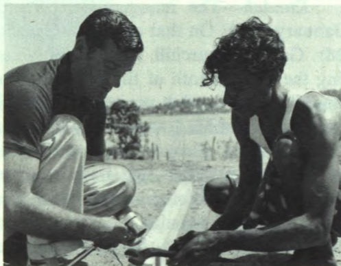
A Canadian expert and his helper working on transmission line towers in Ceylon.
