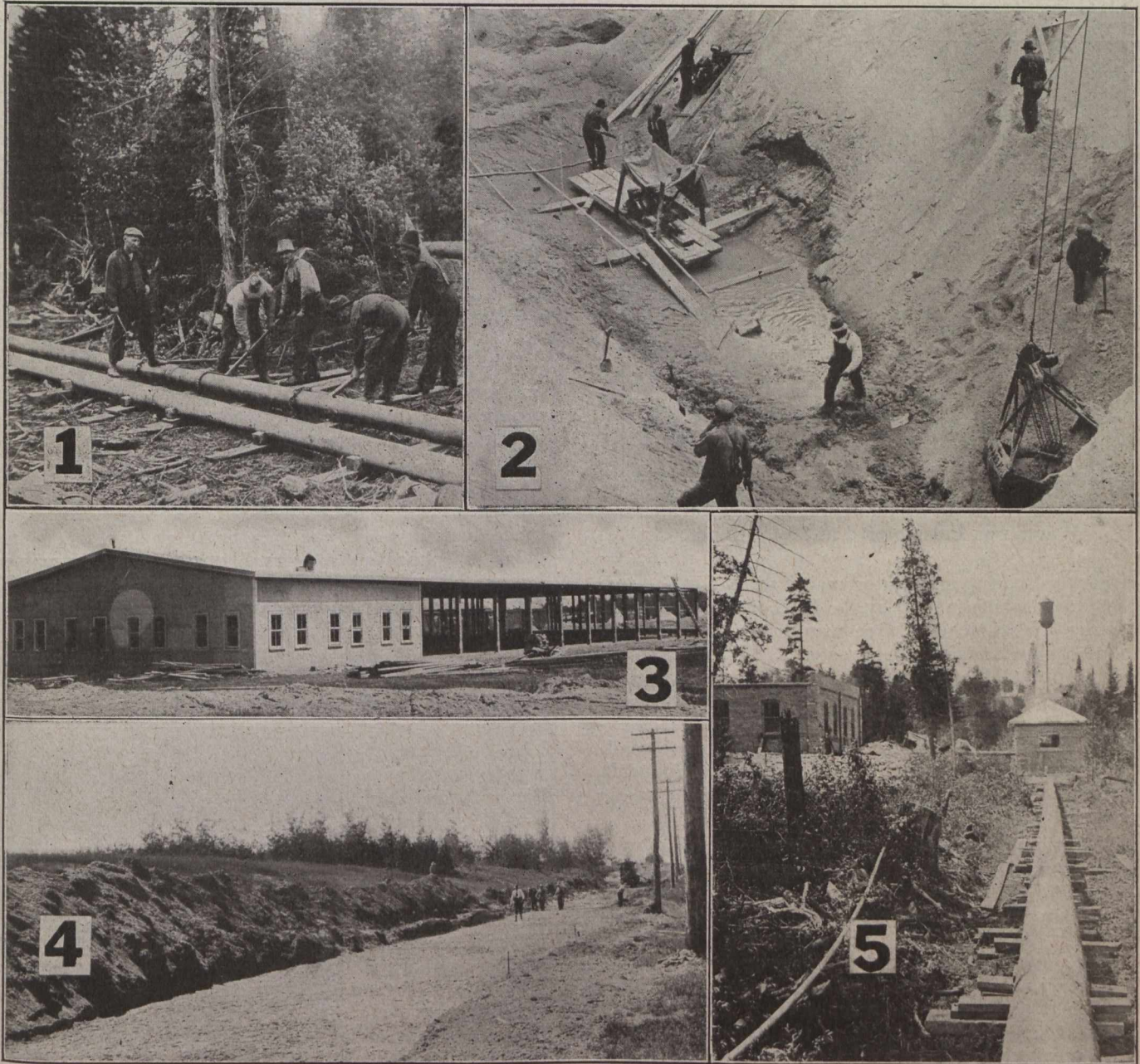
(1) Laying 8-inch Discharge Mains from Pumping Station to Water Tower; (2) Pumping Out Water and Excavating Sand at Site of Sewage Disposal Plant; (3) The Military Garage; (4) Preparing Sub-grade for Concrete Road; (5) View Along Wood Stave Pipe Leading from One of the Wells, with Pump Well and Steel Water Tower in Background, and Pumping Station to the Left of the Pump Well.
