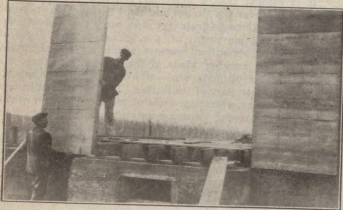
FIG. 1—ONE MAN CAN RAISE PANELS—NOTE THAT FLOOR BEAMS EXTEND BEYOND 2 BY 6-IN. PLANK
