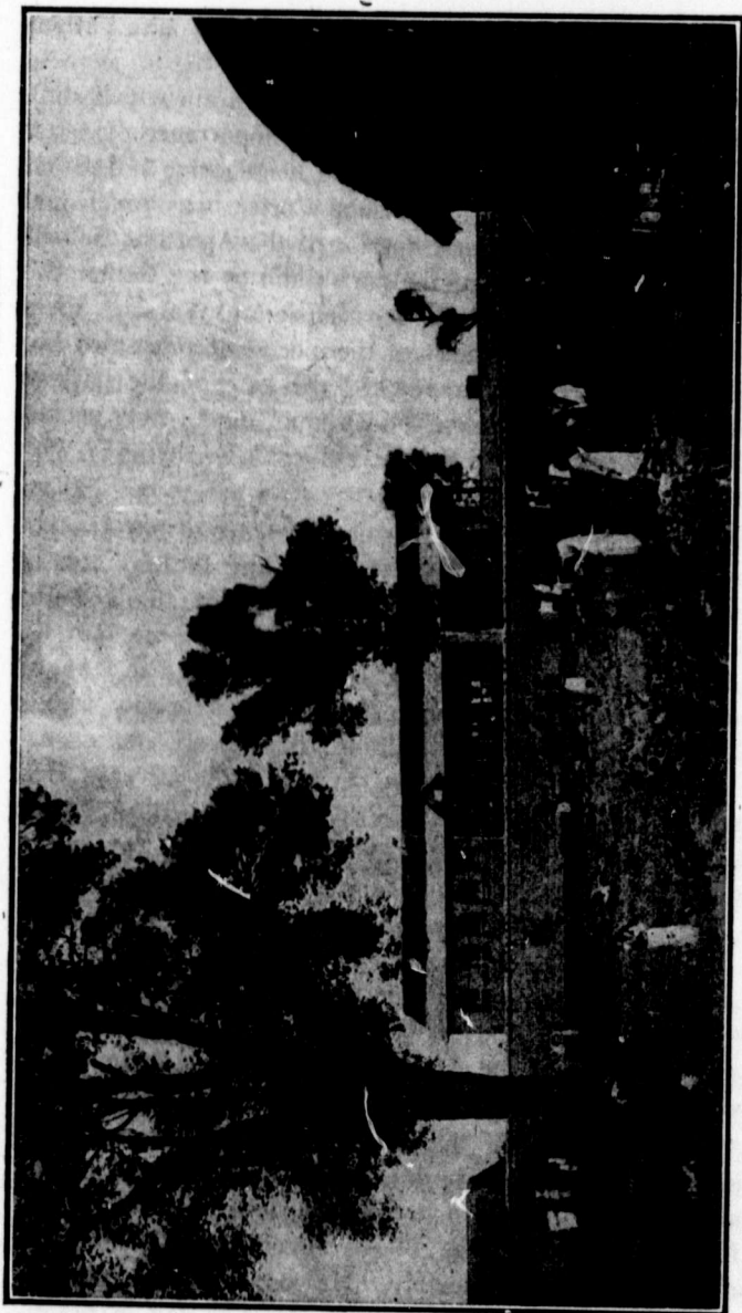
MISSION OF CHILUBULA.—One can see the verandah of which a column gave away, carrying in its fall a part of the upper story.
