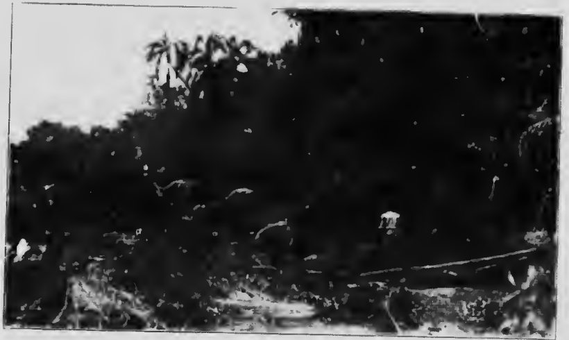
CONSTRUCTING A BRIDGE ACROSS ONE OF THE NUMEROUS CHANNELS OF THE MARA RIVER SEE PAGE 155
