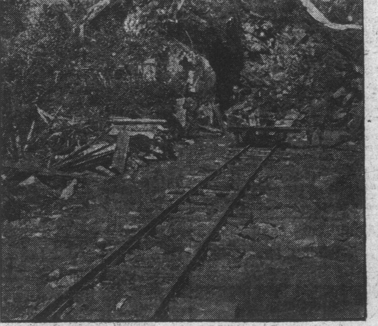
PRINCE RUPERT. The above shows the first cut on the G. T. P. at Prince Rupert. The grade is now 200 feet long and the face of it cut is 33 feet deep in solid rock. In wet weather the large tarpaulin rolled up is stretched across the cut to protect the men while muckin'.
