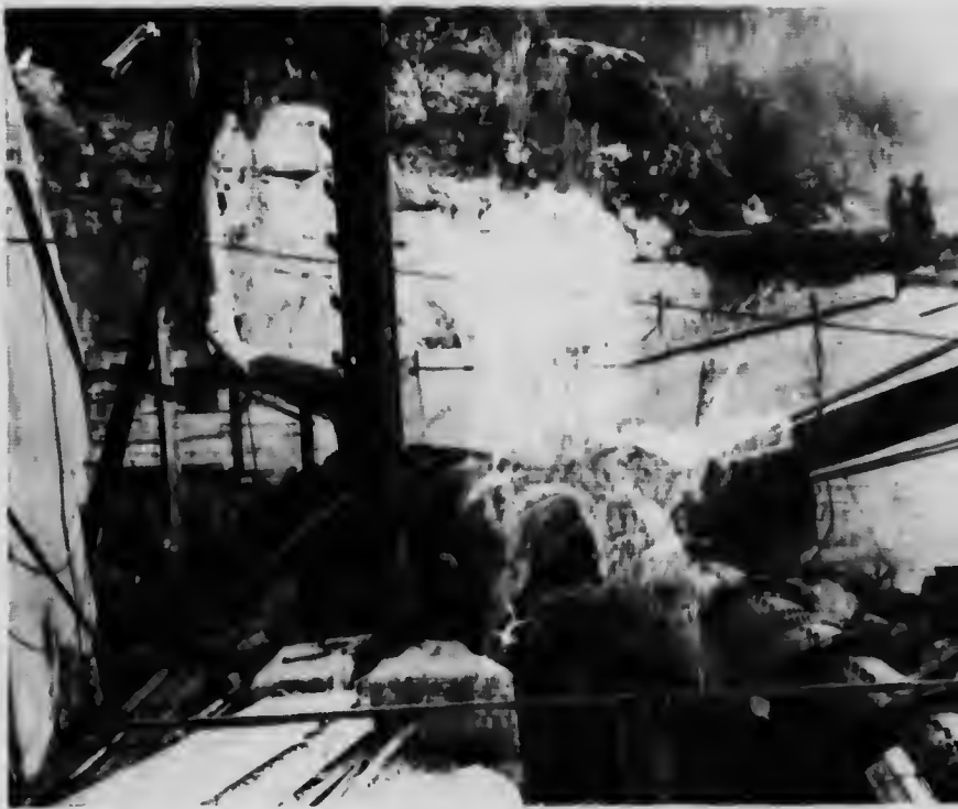
Coquitlam-Buntzen Development. Top of pipe line grade showing No. 1 pipe line with standpipe. Plant No. 2, Lake Buntzen.
