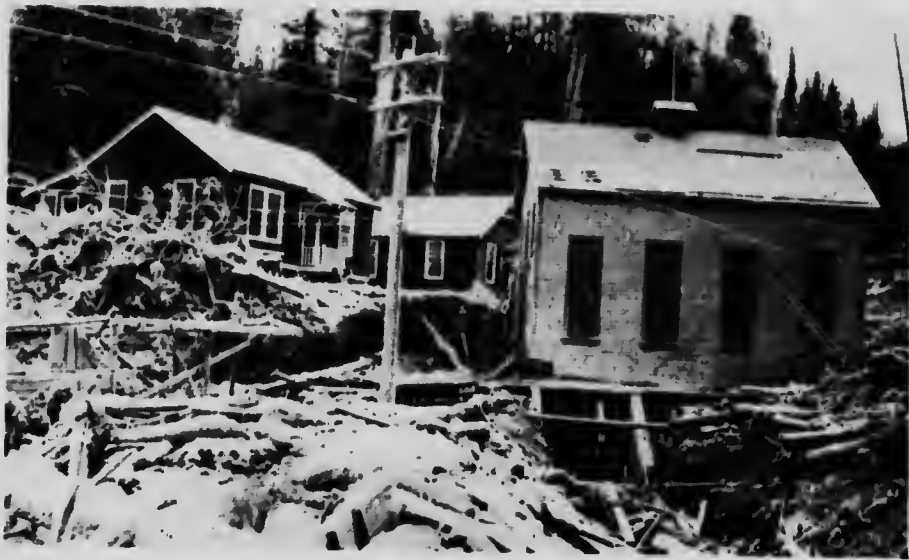
City of Prince Rupert-Woodworth Lake, near Prince Rupert. Front view of Power House.
