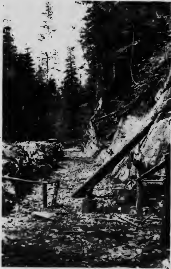
City of Prince Rupert-Woodworth Lake, near Prince Rupert. Grade for 45 inch Pipe Line.
