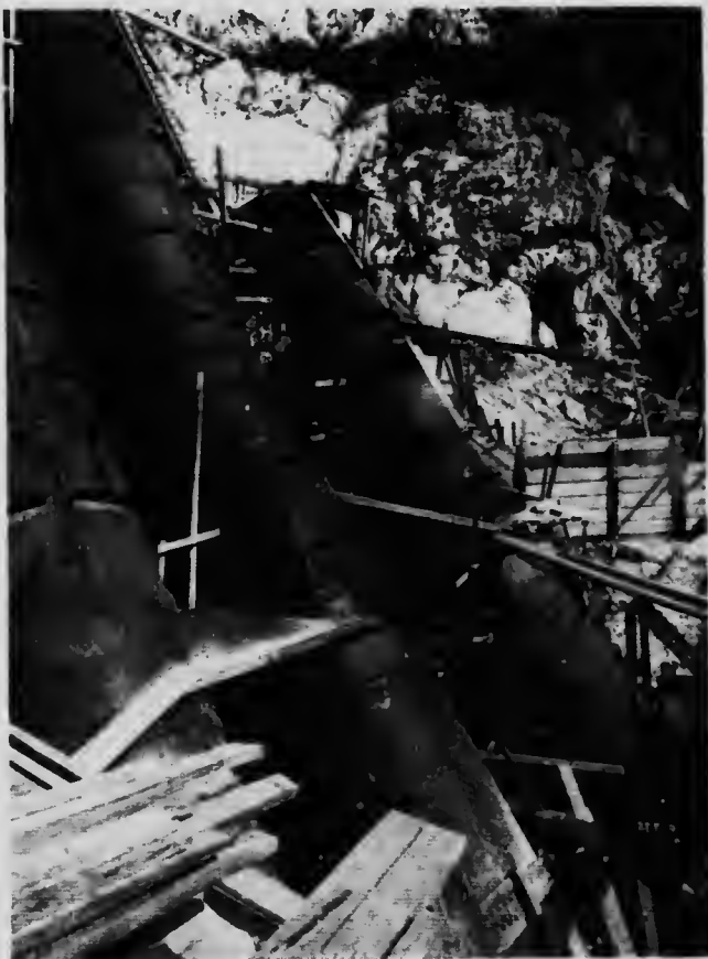
Coquillam-Buntzen Development. Pipe Lines Nos. 1, 2 and 3, Plant No. 2, Lake Buntzen.
