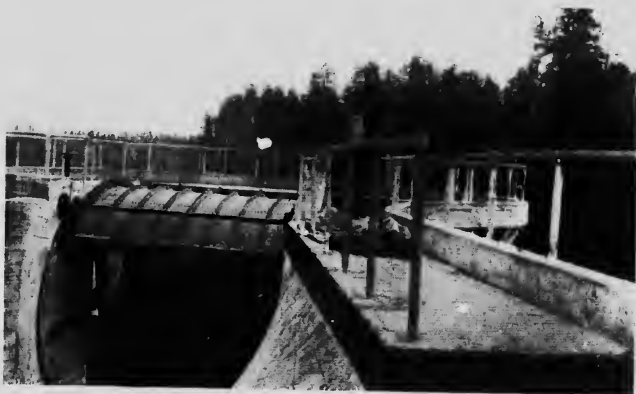
Canadian Collieries (Dunsmuir) Ltd. Fore-bay, showing Screens and Tainter Gate in open position.
