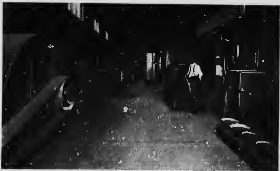
British Columbia Electric Railway Company, Limited. Transformer and Switch Room, Goldstream Power House.
