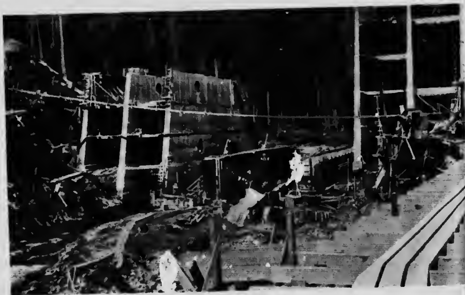
Vancouver Island Power Company Limited. Upstream showing portion of Jordan River Dam in river bed, in course of construction.
