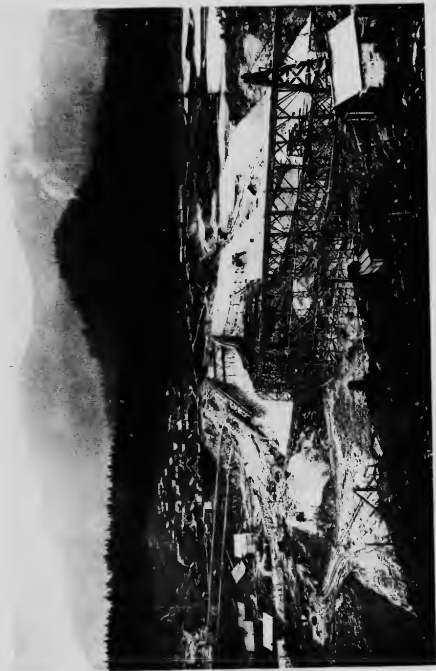
Coquitlam-Buntzen Development. View taken from East Side of spillway showing Coquitlam Dam in construction. The trestle work carries the flume which transports the altered material to the settling pond seen in the middle of the picture.
