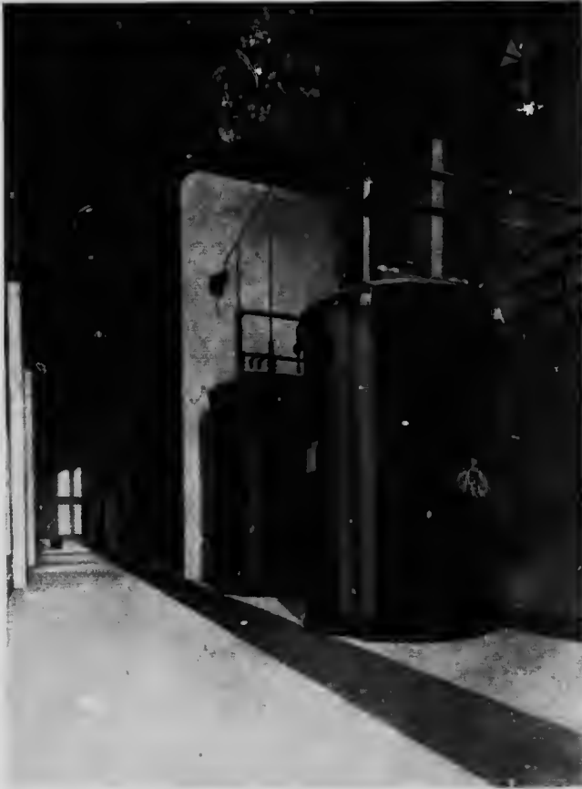
Coquitlam-Buntzen Development. Transformer Room, Power House No. 2, Lake Buntzen.
