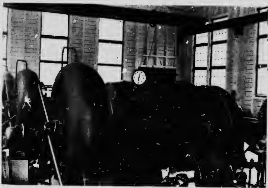
Ocean Falls Company Limited. Interior view of Power House showing Hydro-Electric Units.
