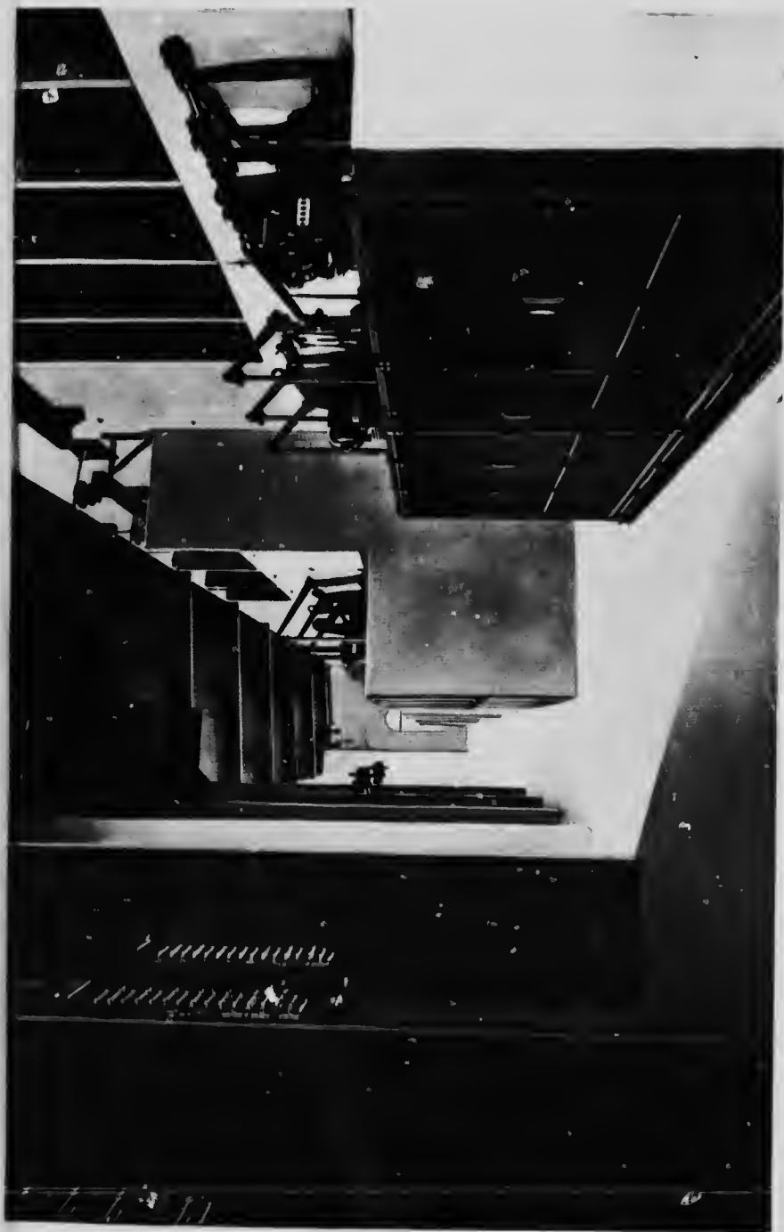
Kootenay River Development. 20,000 and 60,000 Volt Switch and Lightning Arrester Compartment, No. 2 Power House
