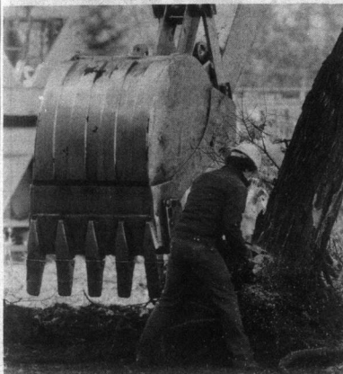
Workers begin ripping out trees in the Arts quad to make way for the new building.
