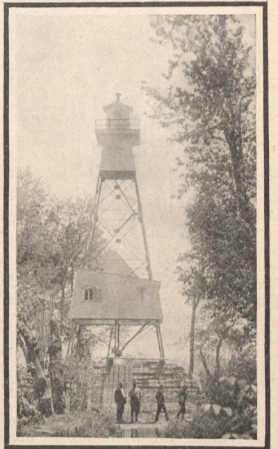
Skeleton Steel Tower on Ile Aux Raisins, St. Lawrence. Here great height was necessary for a back range light.
