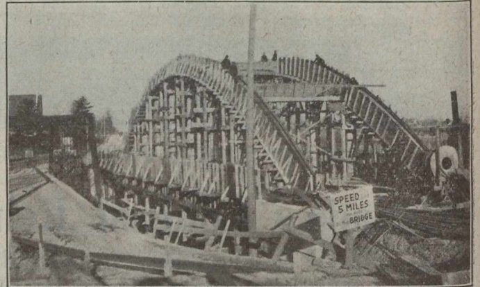
FORMS BUILT, READY FOR PLACING THE ARCH STEEL, BRONTE BRIDGE—OLD BRIDGE TEMPORARILY MOVED TO LEFT TO CARRY TRAFFIC
