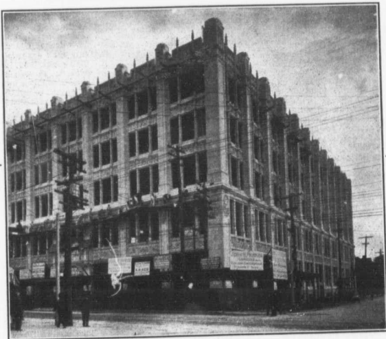
The New Methodist Book and Publishing House at Queen, John and Richmond Streets, Toronto as it appeared on Thanksgiving Day, October 12th.
