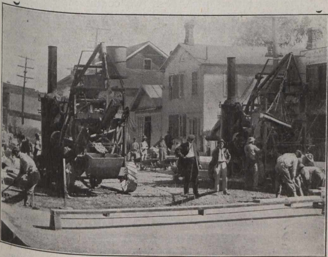
Austin Mixers Working Side by Side on Main Street, Oakville. Roadway, 50 ft. Wide. Full Width of Pavement Carried Forward at Once.
