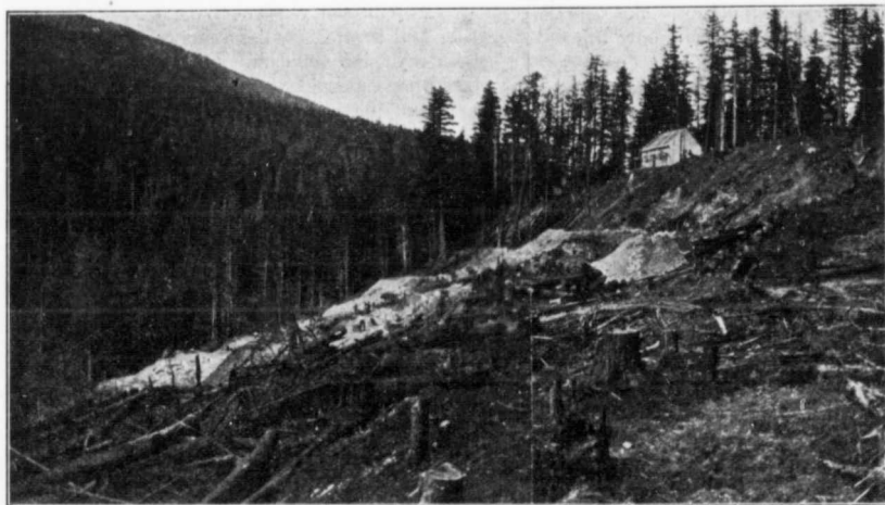
View taken from New Silver Cup tram right of way of upper part of grading for mill site. Blacksmith shop at top of Bend.
