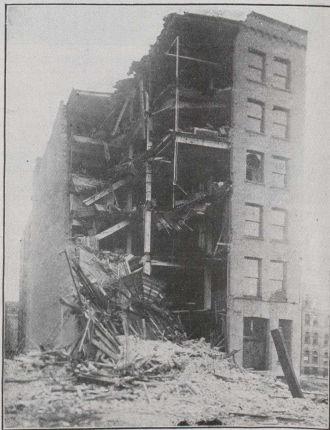
A Six-storey Brick Warehouse, Winnipeg, Manitoba, which Collapsed on July 26th.
