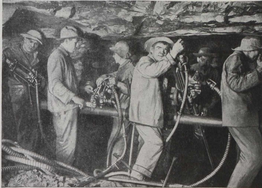
Fig. 6.—Sullivan Liteweight (2½-in.) Rock Drills on an 11-ft. heading bar in the Mount Royal Tunnel
