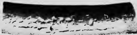
Fig. 1,726. — Corroded Lead-sheathed Telephone Cable Run Below an Electric Tramway.
