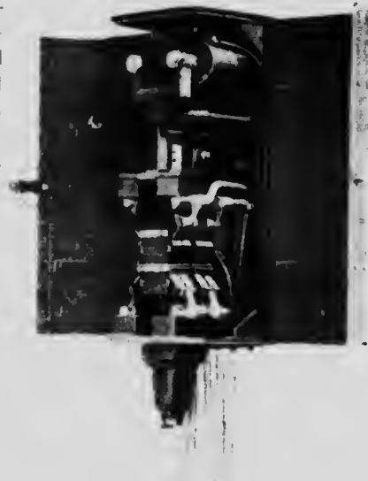
Fig. 17. A view of the contactors in position.
