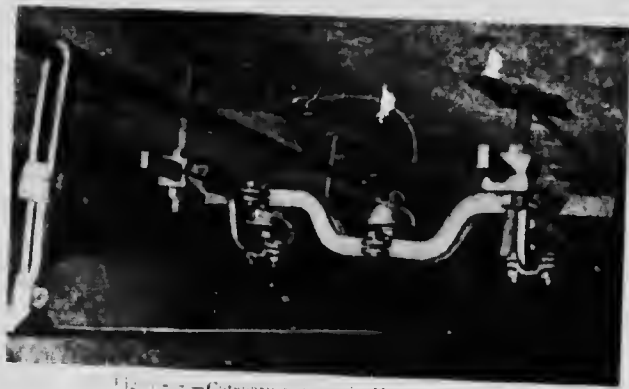
Fig. 1.705.—Catenary Support in Montreal Tunnel.
