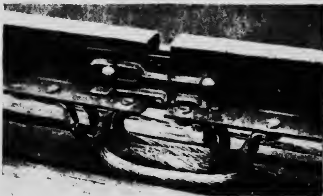
Fig. 1761. Expansion Joint and Bonds on Conductor Rail.
