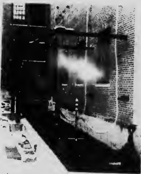
Fig. 1,620. Water Rheostat at Generating Station for dissipating excess Regenerated Energy.
