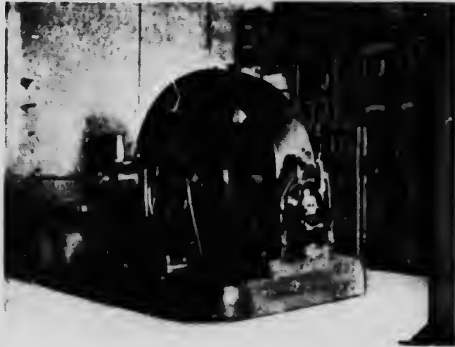
Fig. 103—Interior of a Power Automatic Sub-station
