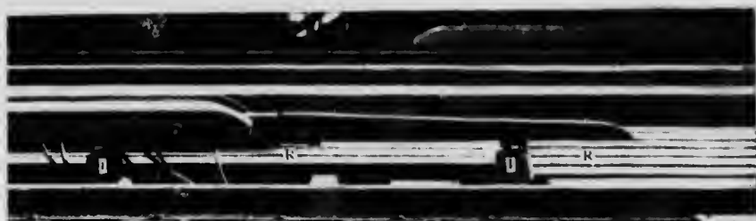
Fig. 1994.—End of Conductor Rail at a Break.
