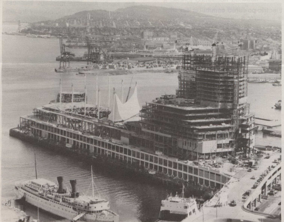
The steel framework for Vancouver's $137-million convention complex was completed in early July of this year.
