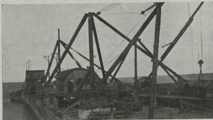
Rock Loading Plant at Point Du Chene.
