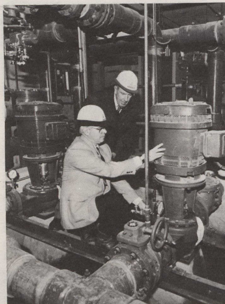
Al Hendry (front) and John Doull examine the pump of the cooling system installed in Halifax, Nova Scotia's new commercial complex, Purdy's Wharf.
