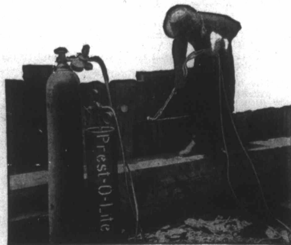
Cutting \frac{3}{8} inch Sheet Steel Piling (including lock joints \frac{2}{4} inches thick) by the Prest-O-Lite Process.
