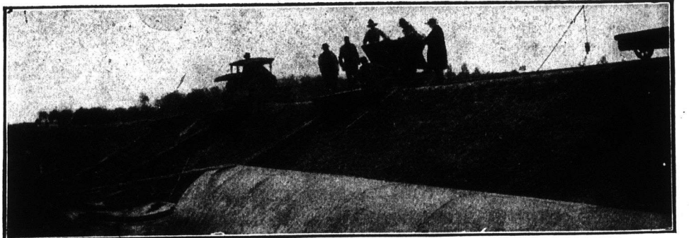
At Work on Winnipeg's Waterworks In the above picture men are depicted in the act of pouring concrete from a wheeled vat through a long pipe into the bottom of the pipe excavation. The vat stands on a narrow gauge railway, of which there are great stretches all along the line of the aqueduct. This railway is used for the carrying of material to the various points where actual construction is being done.
