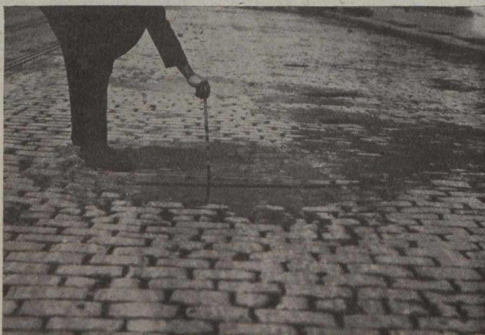
Showing Character of Depression to Pavement.
