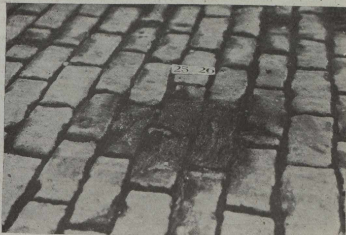
Showing Damage to Granite Blocks.
